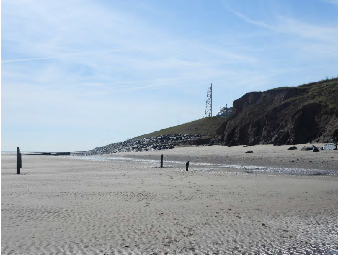
Insert A7-3-7 – Sea Defence and Groyne Structures toward the Southern Extend of the Survey Area at Easington
